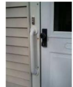
Vertical Grab next to Door
